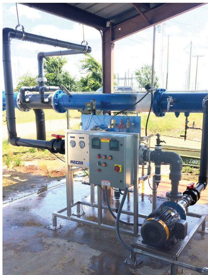
In a system compact enough to mount on a small skid, Mazzei constructed a highly efficient aeration system with a sidestream pump, venturi injector and controls, and includes a Pipeline Flash Reactor. The system raises dissolved oxygen in treated water by more than 60 percent to exceed mandated levels.
