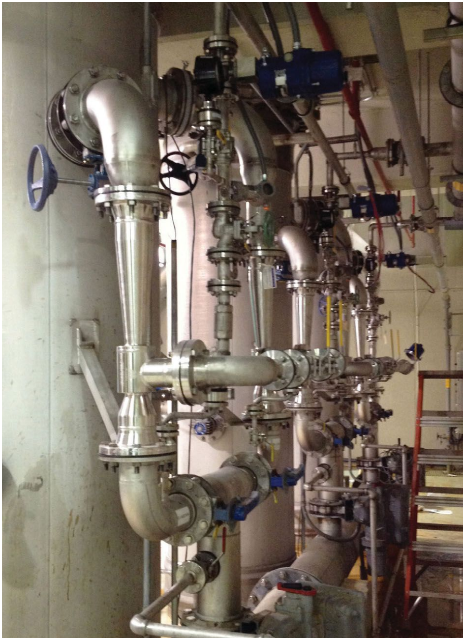
Venturi injectors, like the ones at this treatment plant, are extremely efficient at injecting ozone into wastewater and have no moving parts.
